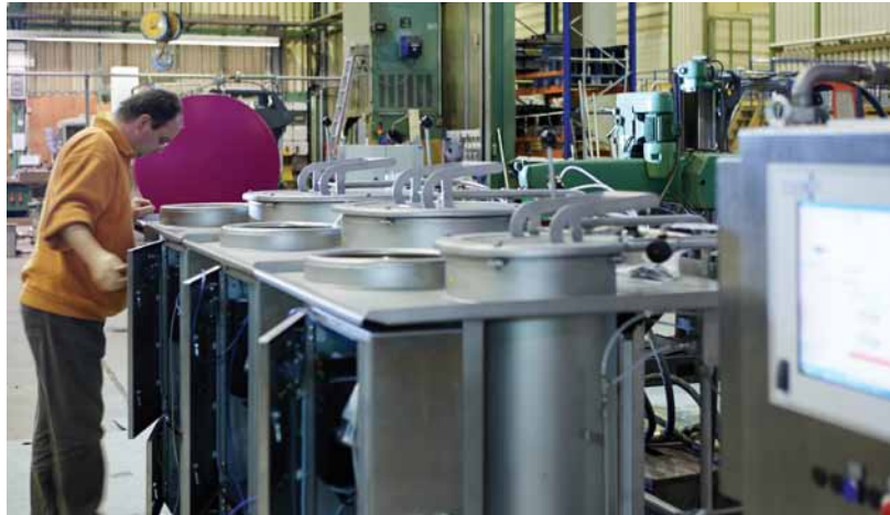
Automatic dosing station for dyes: the dye is mixed and pumped through a system of pipes when needed.
